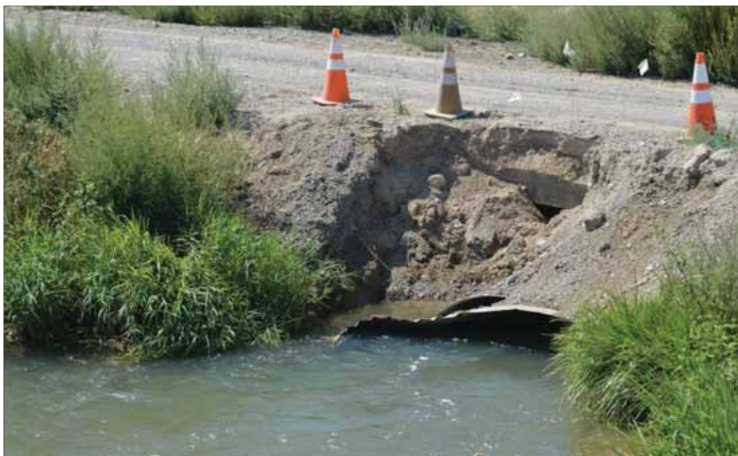
The road surface crossing South Canal is eroding on the east side of Johnstone Road, which has been closed south of Homedale until a new culvert can be installed.
