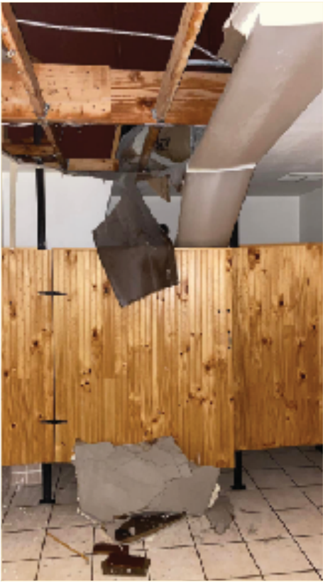
Storm water that had accumulated on the Owyhee County Historical Museum roof came crashing through the ceiling in the front of the building, causing damage in — among other places — the restroom. Submitted photo
