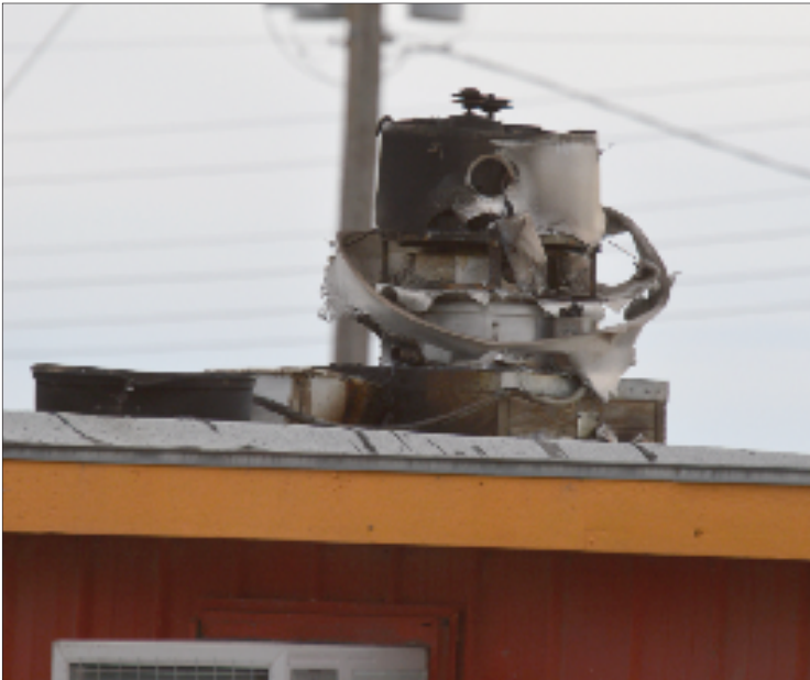
The charred kitchen vent the morning after last Wednesday’s fire.
