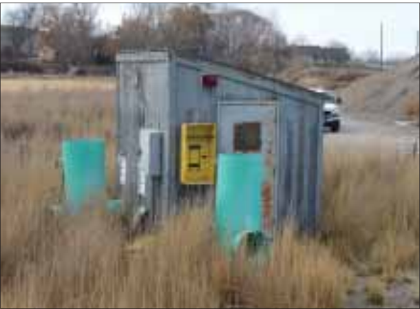
New regulations lowering the amount of chlorine allowed to treat contaminants in wastewater is one reason Homedale is looking at upgrades. This building is where chlorine is monitored at the sewer lagoons.
